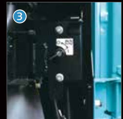
Battery shut-off switch
